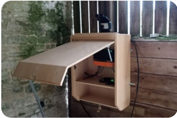
Mains energiser in barn
